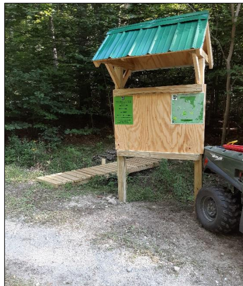
Kiosk and bridge built for the new Hawks Pass trail at Raptor Lane
